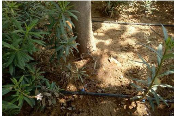
Storm water drain and Drip Irrigation
