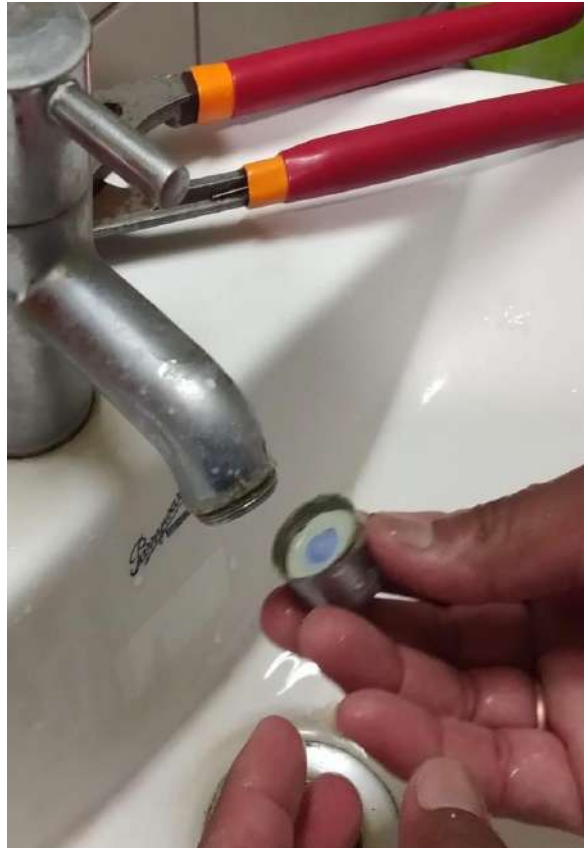
Water Aerator Installed in all Taps for handwash
